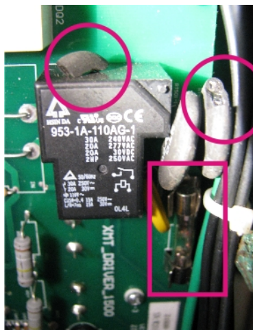
Fig. 26.5: “Exploded” capacitor and burned 30 A / 220V fuse (see rectangle) on Grizzly's controller board for G0722R heavy-duty
